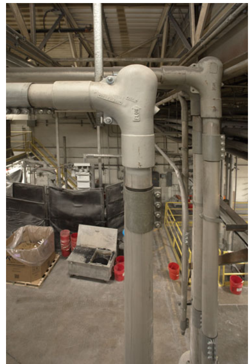
Rhe Tech has only replaced six elbows since installing the original 140 units years ago.
