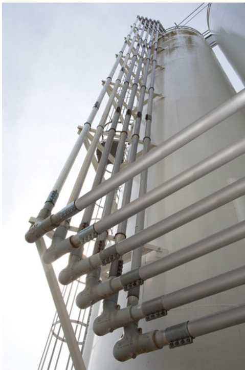
Rhe Tech installed 140 90° deflection Smart® Elbows, preventing blowouts and associated costs of parts, labor, downtime and pellet degradation.
