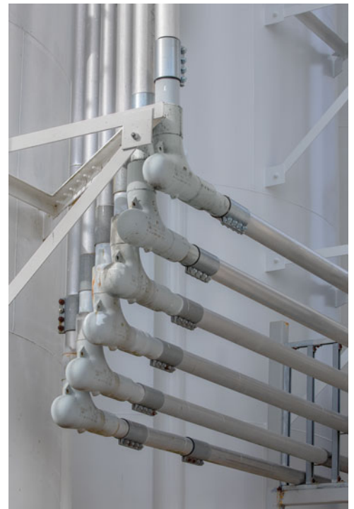
Pneumatic lines transport glass-fiber reinforced pellets to 100 silos and truck stations. Conventional stainless steel long-sweep elbows had been blowing out once a month per elbow and were damaging pellets.
