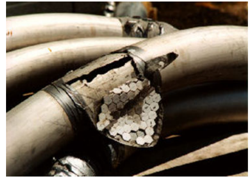
A common sight at RheTech before the HammerTek Smart Elbow deflection elbows were installed was an attempt at patching with ceramic tiles and duct tape.
