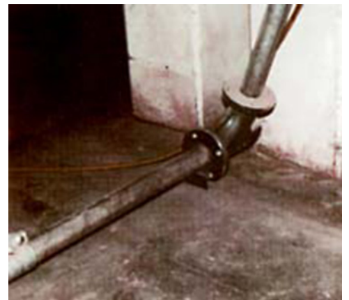
FIGURE #2: The HammerTek Smart Elbow deflection elbow sends "fines" from a line on the floor upwards to the cyclone. These fines are small food particles which are later recycled back into the production line. The upper end of this vertical run is shown in figure 3.
