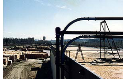
The first Smart Elbow model installed at Northwood in the hog fuel conveying system (above) worked so well that the two sweep elbows also shown above were eventually replaced with two more 12 in. cast iron HammerTek Smart Elbow models.
