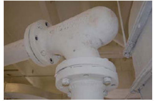
This HammerLoy™ Series Smart Elbow deflection elbow from HammerTek, Bethlehem, PA, is one of 14 such elbows installed at the upper Occoquan Water Reclamation Plant in Centreville, Va. To eliminate pipe failures in the conveying line. After more than four years in operation, all of the Smart Elbow deflection elbows continue to perform as specified without a single pipe failure.
