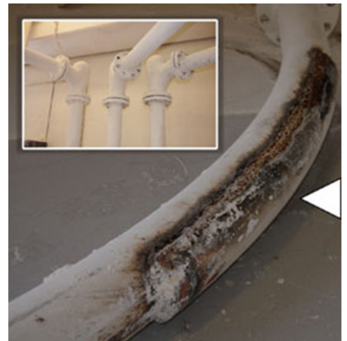
This sweep elbow is one of many that failed to handle the abrasive pebble lime used in the treatment process at the upper Occoquan Water Reclamation plant in Centreville, VA. Such elbow failures, which caked the facility with lime dust as shown on the floor, were plaguing the facility.
