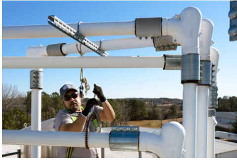
Horizontal sections of pneumatic pipelines conveying abrasive sand are rotated 90 degrees every two weeks to reduce wear.
