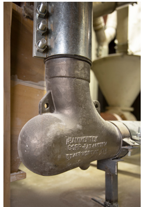
Smart Elbow® deflection elbows solved the problem of sweep elbow failure due to abrasive wheat impacting elbow walls.
