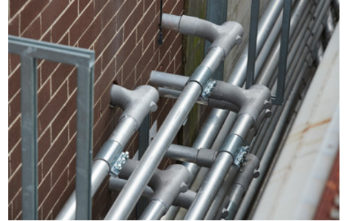
The short radius of Smart Elbow® deflection elbows allows routing of conveyor lines in the restricted space between rail cars and the plant.
