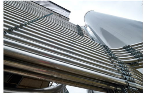
A complex of pneumatic pipelines transports polyethylene resins from rail cars to storage silos and into the plant for processing.
